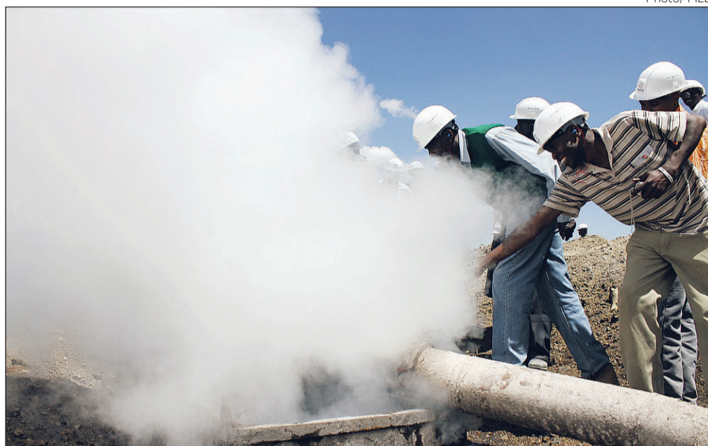
STEAM POWER: Shareholders on a tour of the Kengen Olkaria power generation plants in Naivasha.
